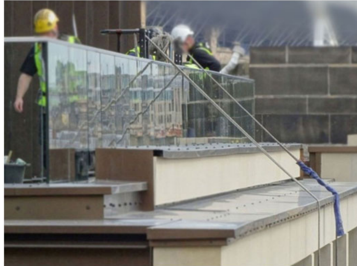
Figure 4 - Anchor device not used in accordance with the manufacturer's instructions. Lack of adequate edge protection (Note: Each rope should have independent rope protection).
