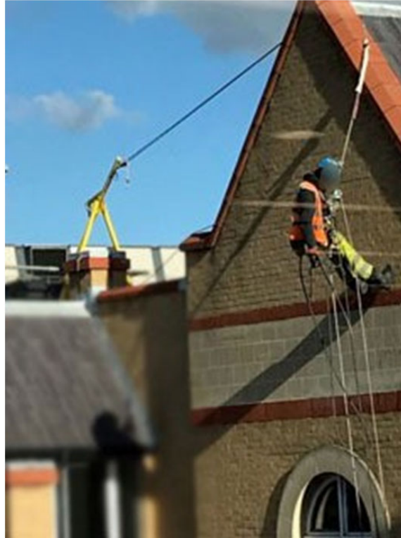
Figure 1 - Use of a placed anchor device outside the manufacturer's instructions. Poorly assessed deviation and rope protection. Rescue complexities.
